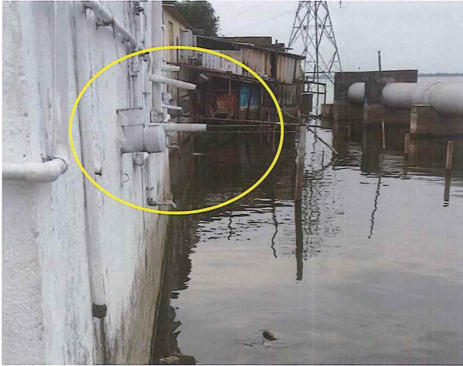
P5 – Sewage outlet from household in Banu Nagar directly discharging into Puzhal lake
