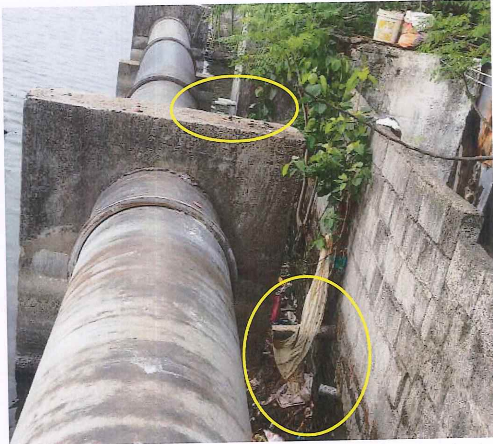
P6 – Sewage outlet from household in Pudur directly discharging into Puzhal lake
